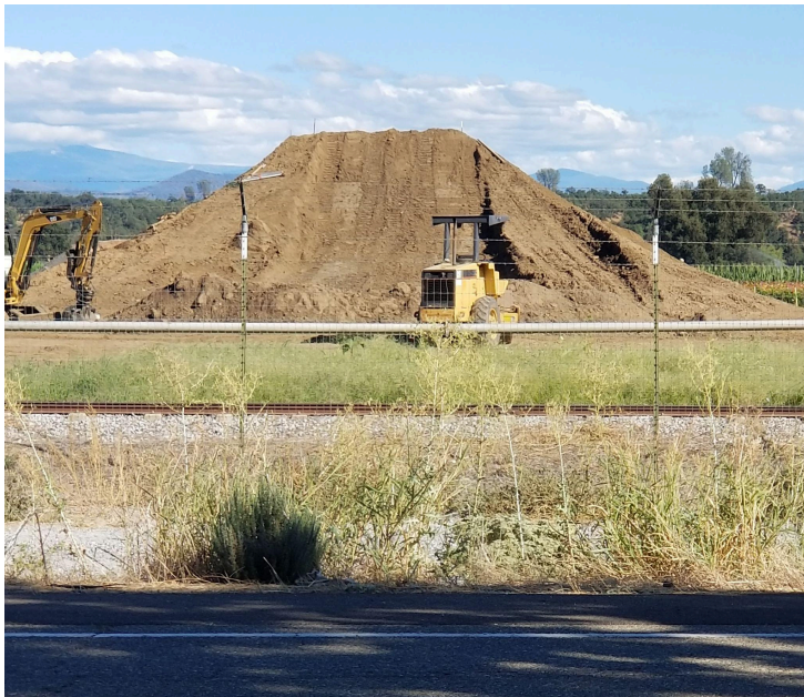
Hawes Ranch - moving dirt to change the landscape. County says no environmental mitigation is required.
